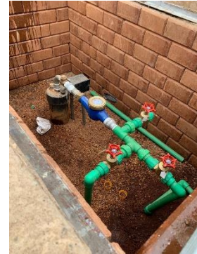
Well pump pit
